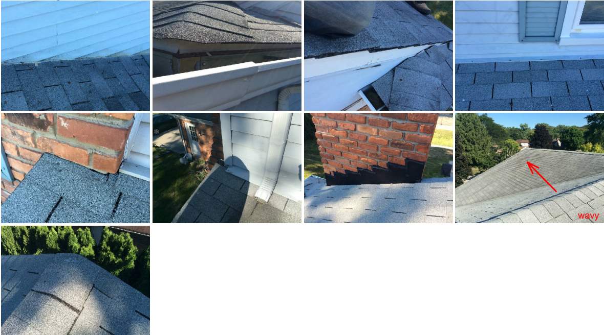
7. Plumbing Vents: PVC - Roof boot is damaged/cracked
